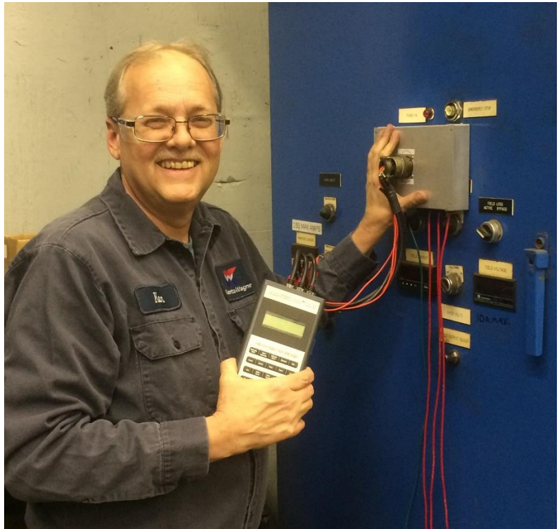
Patterson prepares to install an ALL-SAFE PRO® so he can use an ATPOL II™ to perform energized motor testing.
